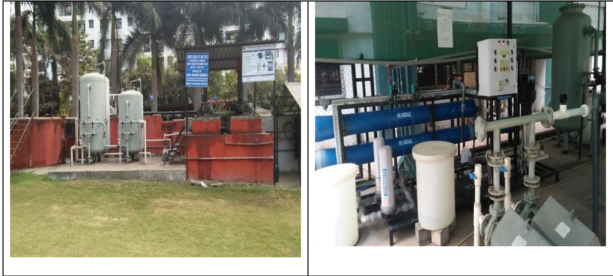
Fig: Sewage Water Treatment Plant in the Campus
